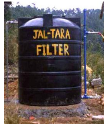
Jal TARA water filter tank.
