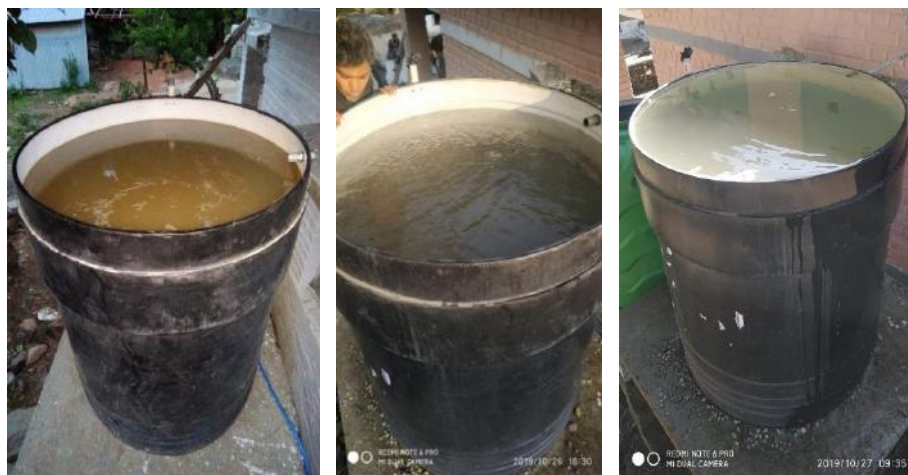
Quality of water in filter tank at three stages- left: after 2 hrs of backwashing, middle: after 6-7hrs of backwashing, right: after 12 hrs of backwashing.
