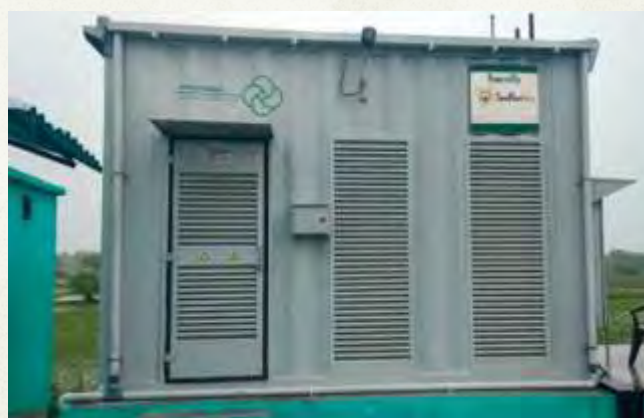
Lithium ion Battery Energy Storage System & Grid-lock, Shivpura U.P
