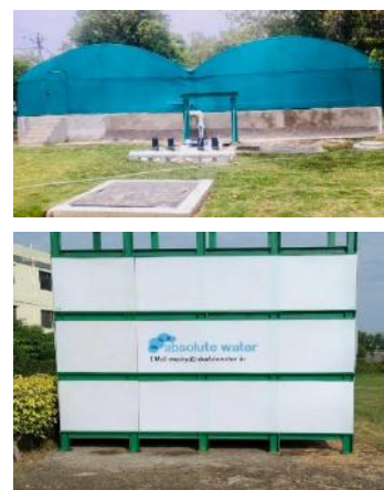
Picture 7 Civil based Bio-STP by Absolute Water(left), Modular Unit(right)
