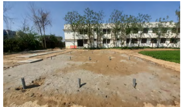
Taisei Soil System / Tafgard technology to treat wastewater discharged from hostels implemented at Shri Ram Group of College, Muzaffarnagar Campus.
