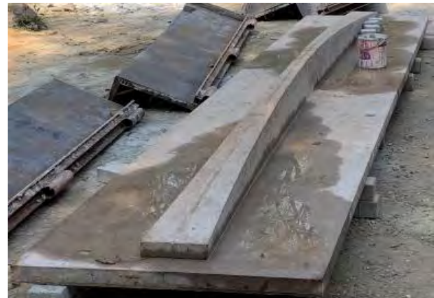
Experiment conducted in Ghitorni, New Delhi to develop a structurally optimized roofing product using LC 3
