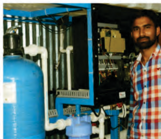
Water Treatment Unit
