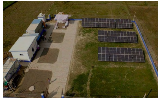
TAR Aurja solar power plant at Parsa, District Saran, Bihar
