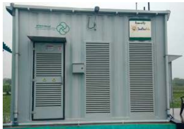
Lithium ion Battery Energy Storage System and Grid-lock, Shivpura Uttar Pradesh
