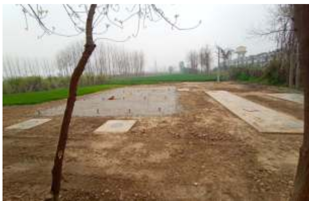
Taisei Soil System technology installed at Shri Ram Group of Colleges, Muzaffarnagar, Uttar Pradesh
