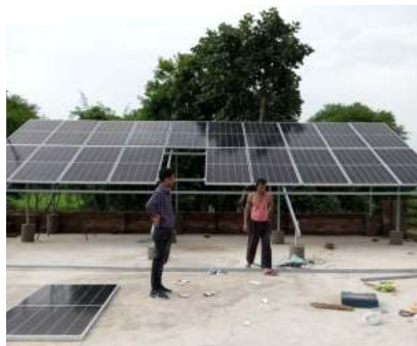
Akash Sahu from Niwadi installing his solar panels for his oil expellers, which saves him INR 3500 monthly by reducing his dependency on fossil fuels
